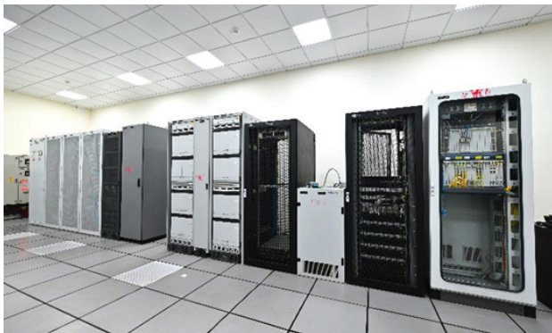
GSMR Server Room at OCC Ahmedabad
