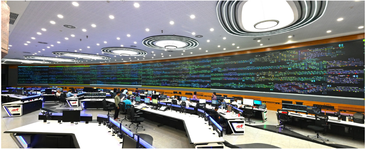
Inside view of OCC Ahmedabad
