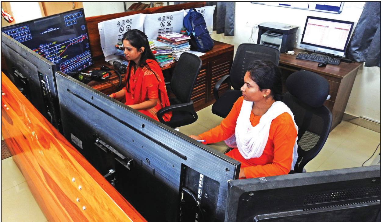
Controlling of Sanand North Station by all Women Staff
