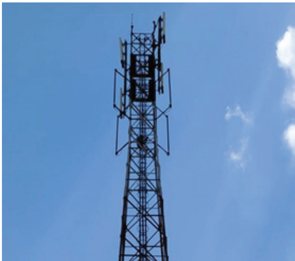
UHF Antenna for Kavach on Tower
