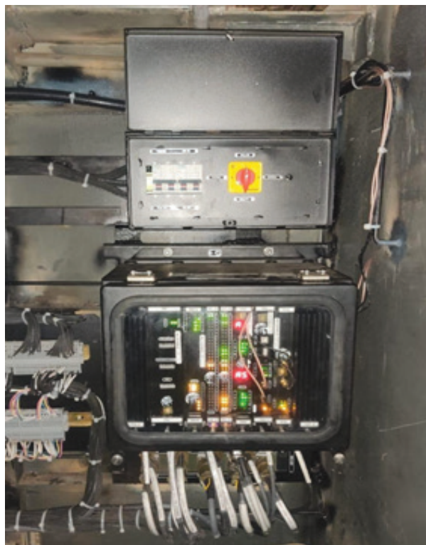
Loco Kavach installed in a Loco
