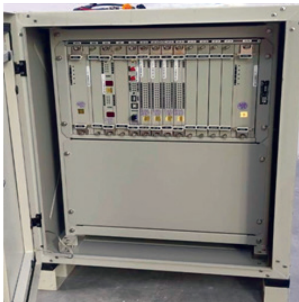
Station Kavach Installed at a Station
