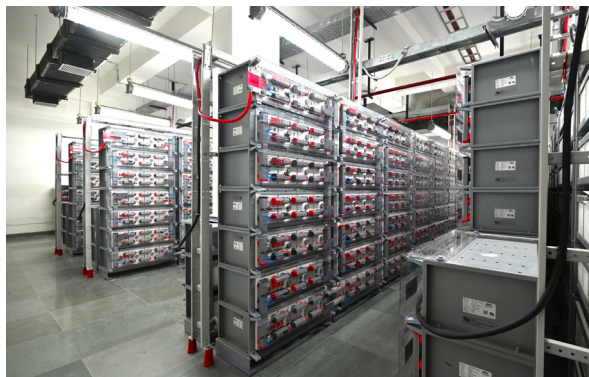
Signal & Telecommunication Battery Room at OCC Ahmedabad
