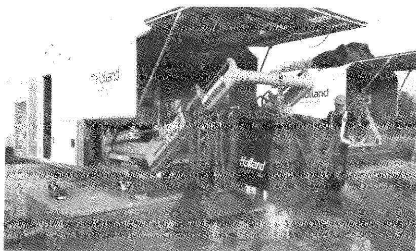
Flash Welding Plant At Bhagega- WDFC
