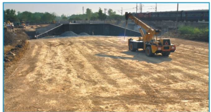
Block filling in progress at A-2 of Bridge No. 318, at km 191/30-32 in Atul-Valsad block section between Bombay Central-Surat station in Valsad District of Gujarat
