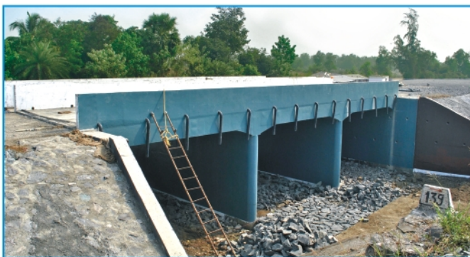
Painting work in progress of Bridge No. 139, at km 96/16-18 in Palghar-Umroli block section between Bombay Central-Surat station in Thane District of Maharashtra
