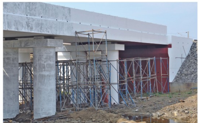
Progress of Bridge No. 119, at km 83/32-84/2 in Kelve Road-Palghar block section between Bombay Central-Surat station in Thane District of Maharashtra.
