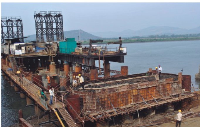
Shuttering arrangement Pile cap P-I of Bridge No. 92, at km 69/2-16 in Vaitarna Saphale Block section between Bombay Central-Surat station in Thane district of Maharashtra.
