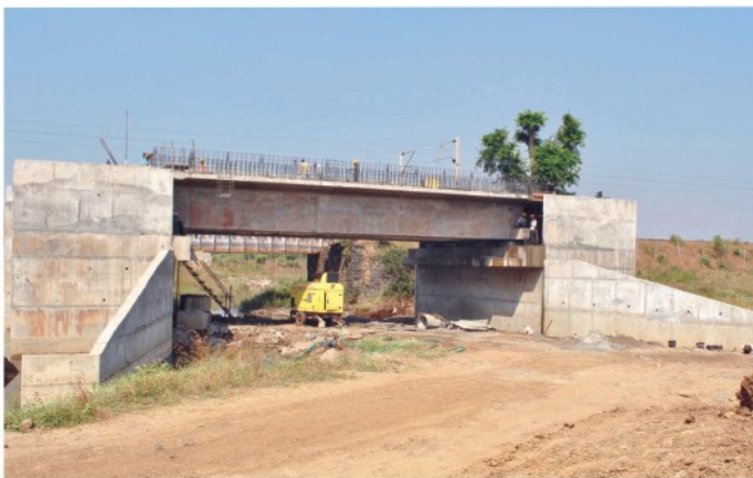
Progress of Bridge No. 239, at km 153/28-30 in Sanjan-Bhilad block section between Bombay Central-Surat station in Valsad District of Gujarat.
