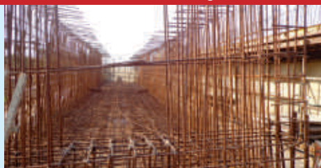
Reinforcement binding is in progress for P5-A2 Up track Box girder at Bridge No. 611, Kymorre (Bihar) between Kudra-Shiv Sagar
