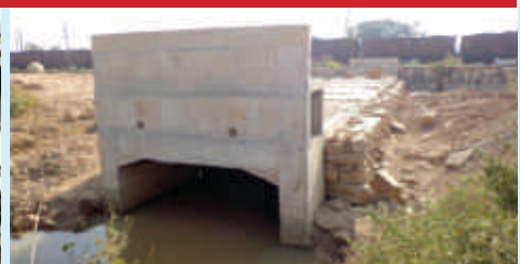
Boulder packing completed at Bridge No. 613 at Kymorre (Bihar) between Kudra-Shiv Sagar
