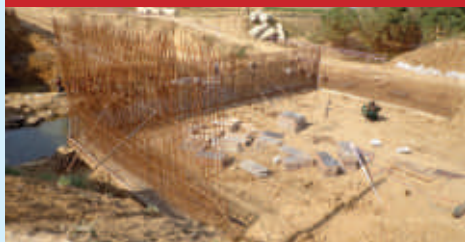
Reinforcement binding is in progress for abutment/wing wall (A-1 location) at Bridge No. 615A at Kymorre (Bihar) between Kudra-Shiv Sagar
